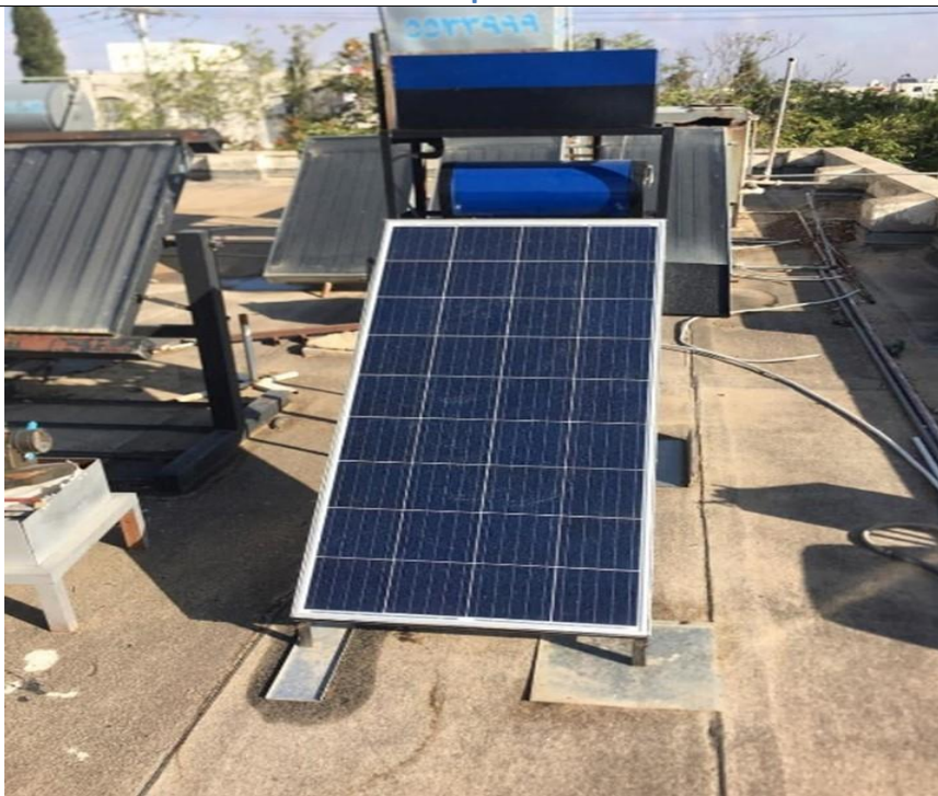
Solar Panels + Solar collector (Thermal energy)
