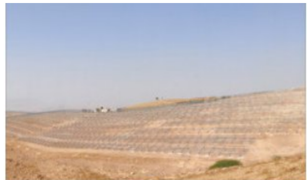
(BAU) solar PV plant
