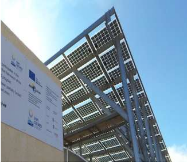
Photovoltaic Solution Package AL-BALQA UNIVERSITY (onyxsolar.com)
